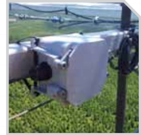
Contractor: Electro Kingsey Products Used: 10 JBX666
