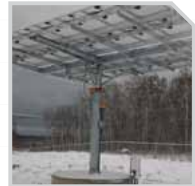
Contractor: Guardian Electric Inc. Products Used: 500+ JBX884 & JBX12124
